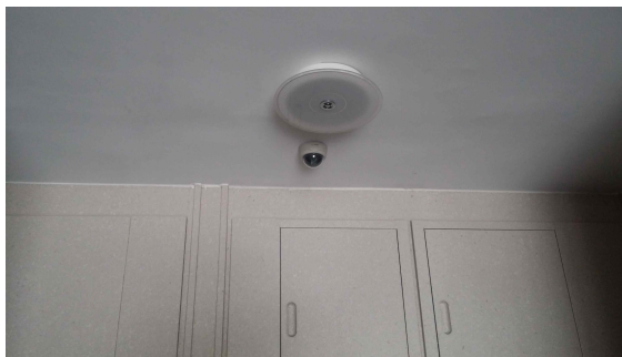
Figure 14. F apa.: CCTV in elevator hall
