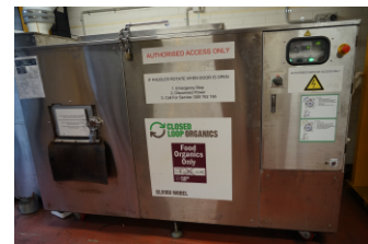
[Figure 5] Organic waste machine (Student Union)
